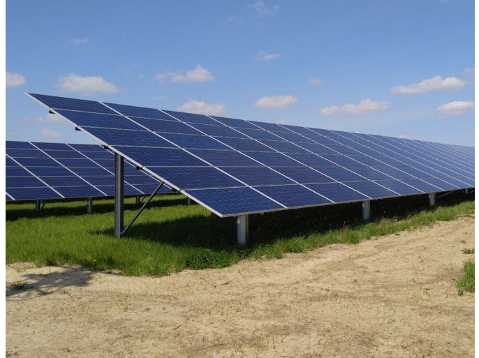
The Village of Minster keeps the grass short at its 4.2-MW solar project by bringing in a herd of sheep in the summer.
