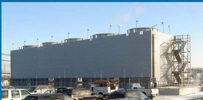
North Cooling Tower
