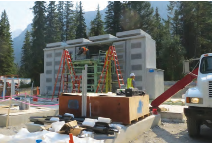
During construction for the battery at Field, the battery enclosure is erected and the modules installed prior to construction of the building.
