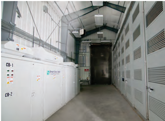
NGK's NaS battery (right) and S&C's SMS (left) located inside the prefabricated building at Field.
