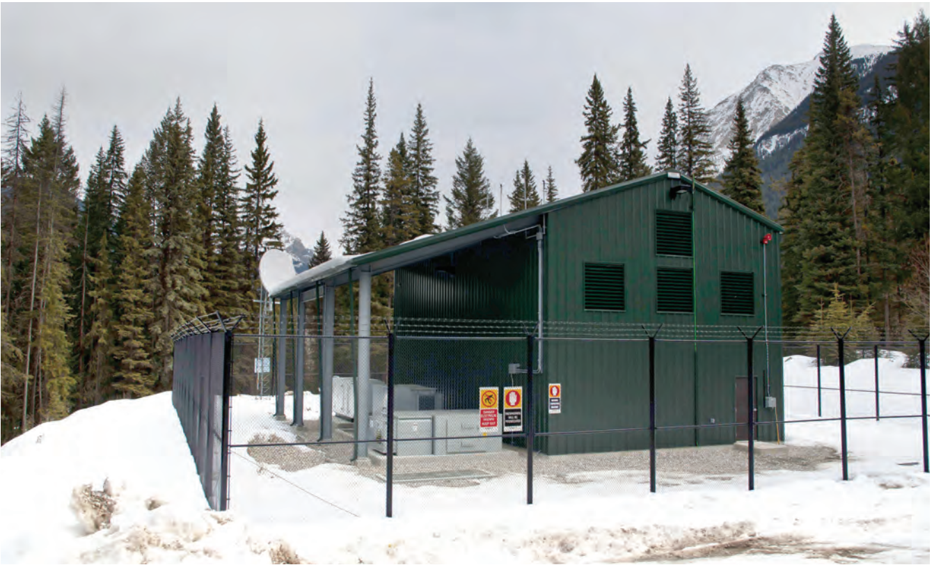
In the mountainous town of Field, Canada, the completed NaS battery energy storage installation went into service in May 2013.
